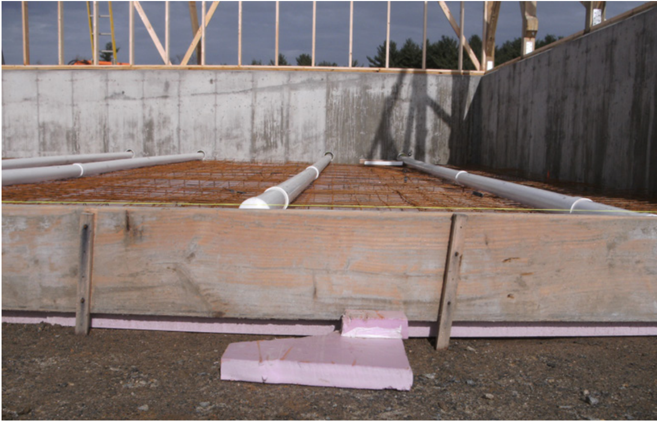
Figure 21: Insulation below Main Composting Floor at UNH Composting Facility
