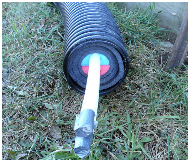
Figure 11: Insulated Underground PEX Pipe used Between Compost Facility and Milk House
