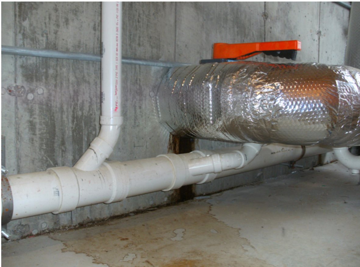
Figure 61: Leak through the Back Push Wall
