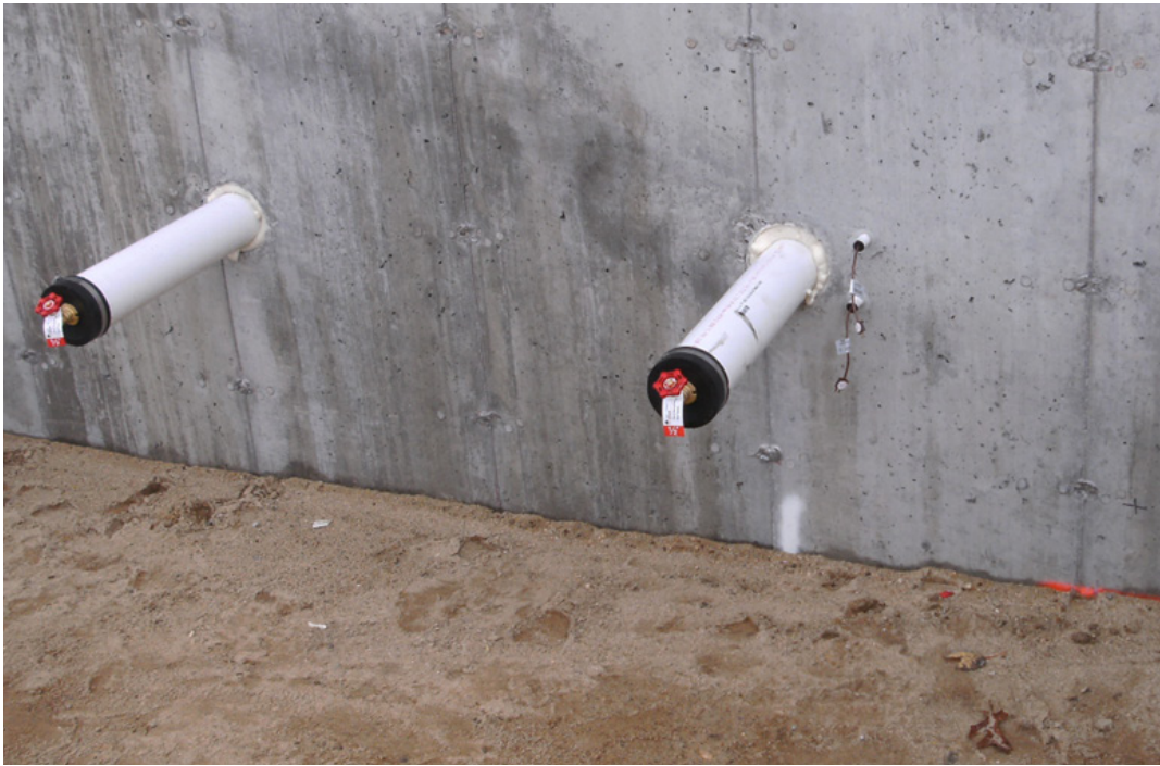
Figure 26: Aeration Lines through Back Push Wall with Hose Bibbs
