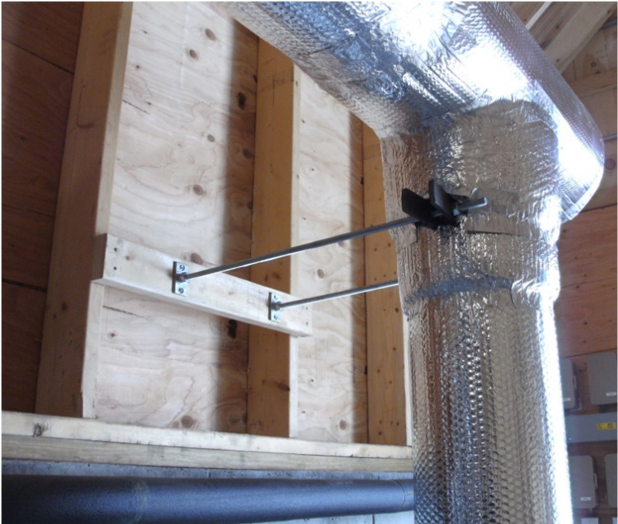
Figure 60: UNH Aeration System Insulated with Reflectix
