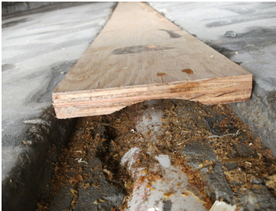
Figure 35: Profile of a Cover Plate over an Aeration Line (Plate yet to be drilled)
