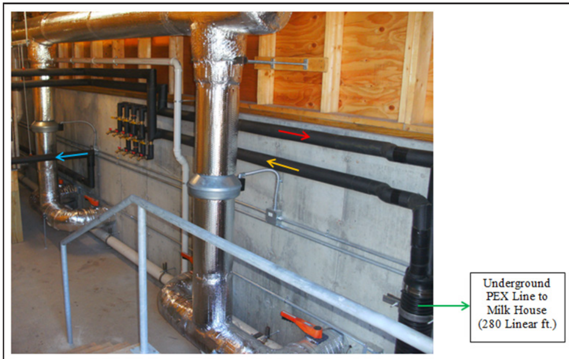
Figure 54: Hot Water Supply and Return Lines in the Composting Facility
