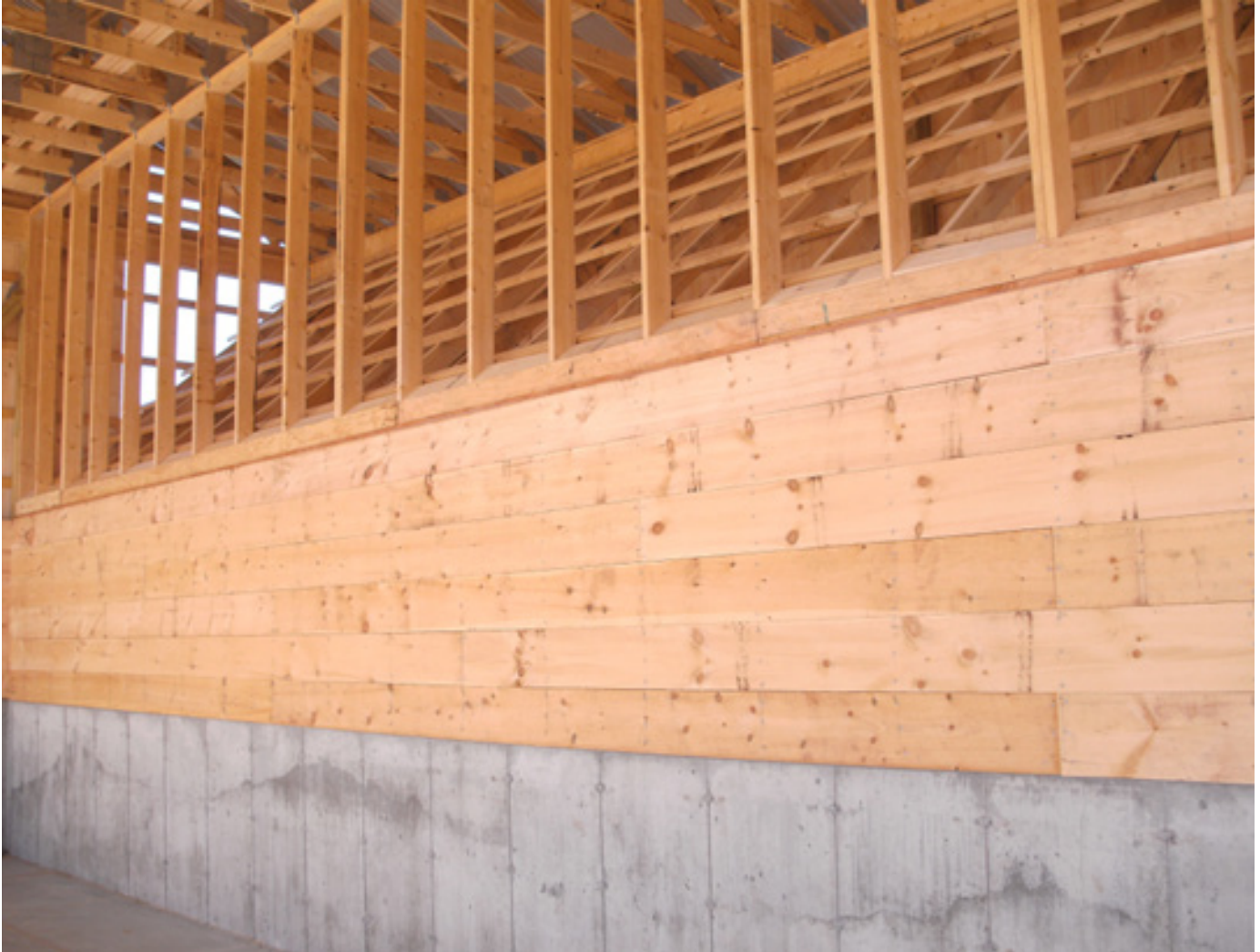
Figure 18: Back Push Wall at UNH Composting Facility
