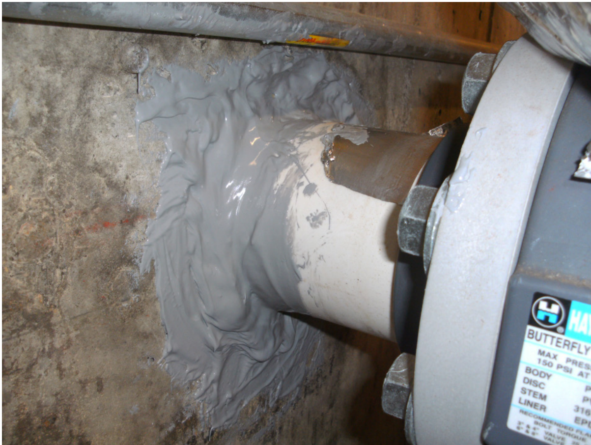
Figure 62: Replacement Expanding Joint Filler on the Mechanical Room Side of the Push Wall
