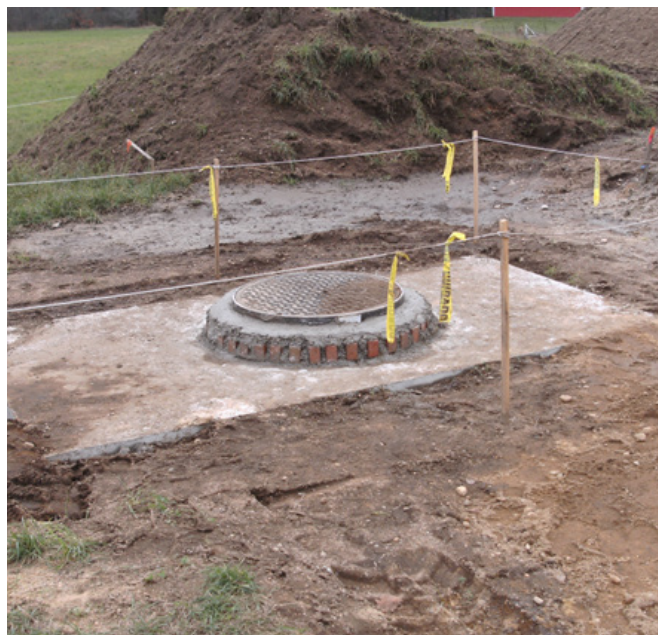
Figure 12: Compost Leachate Tank at UNH Facility
