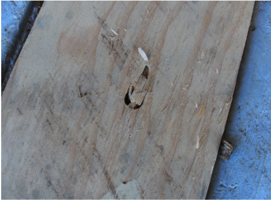
Figure 37: Cover Plate Aeration Hole with Chipping
