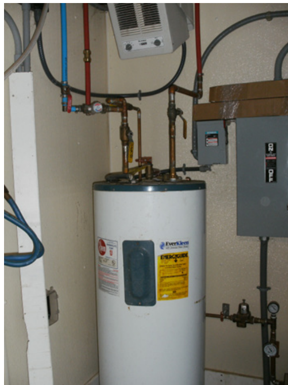
Figure 57: Primary Farm Hot Water Heater Receiving Tempered Water from the Heat Exchange Unit
